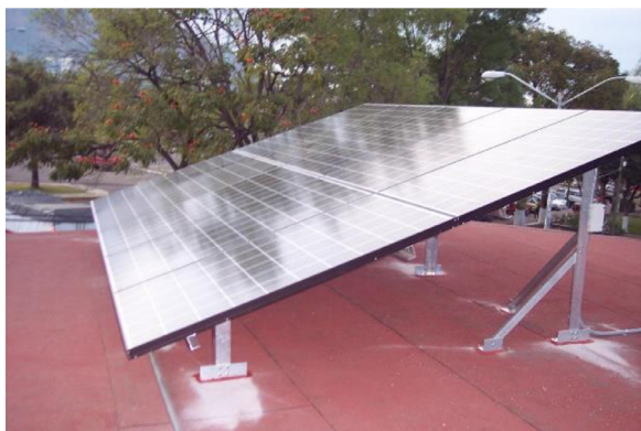
Fig. 4. A 2.4 kW p PV system installed at the roof top of a building of the University of Nayarit, Mexico, installed in the year 2012. The daily production was monitored through an inverter-web-box over 9 years toward 2020.
